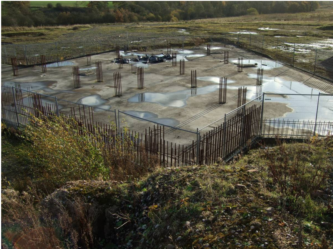
Photograph 8 Panorama of eastern plateau in the northern part of site showing partly built scheme
