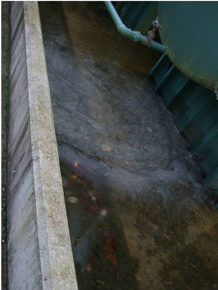
Photograph 16 Oily sheen on water in bunded enclosure below fuel tanks
