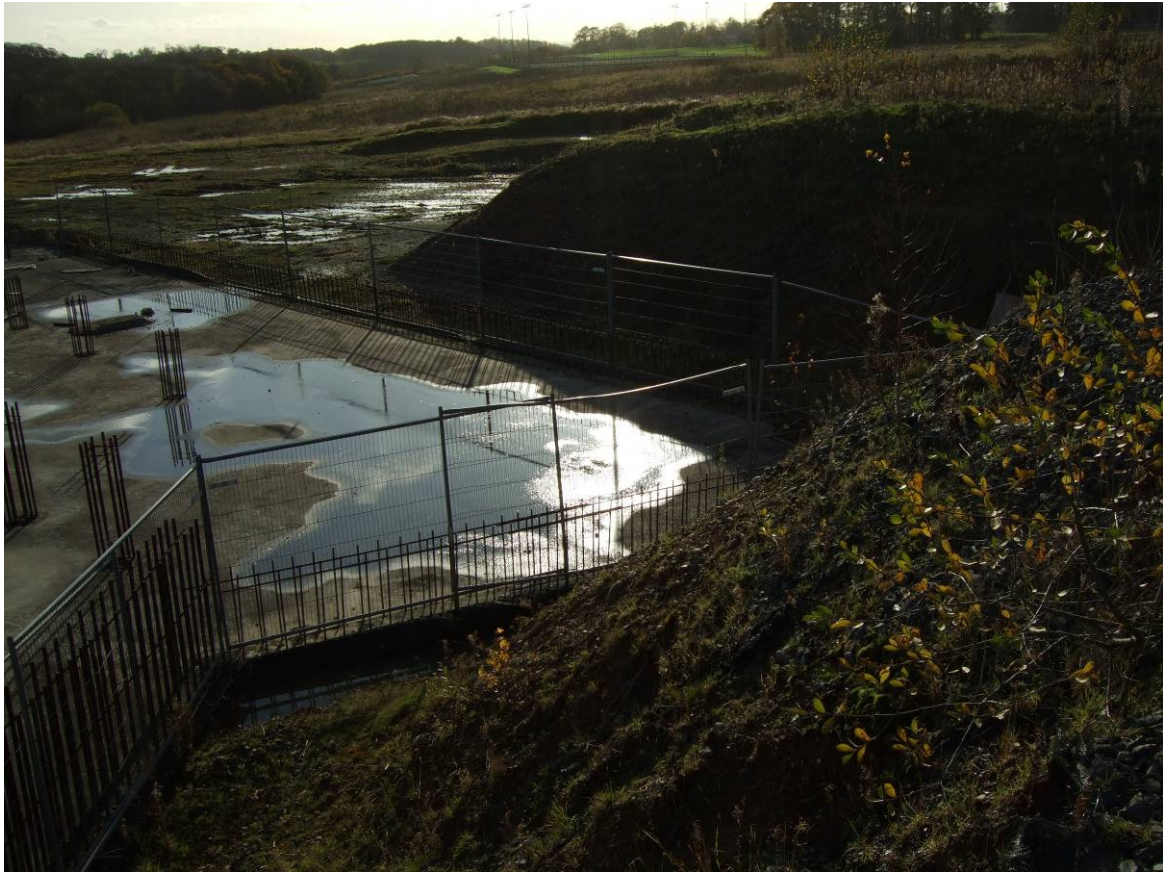
Photograph 9 Panorama of eastern plateau in the northern part of site showing partly built scheme
